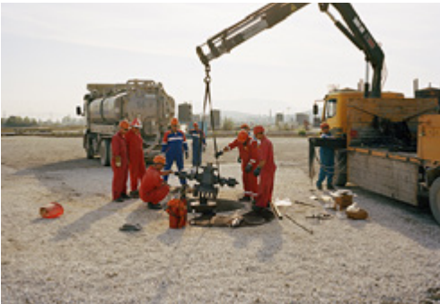
Bankers Petroleum employees install a new well head at the Patos-Merinja central extraction area, Albania, September 2018 (Felix Davey/CAO).
