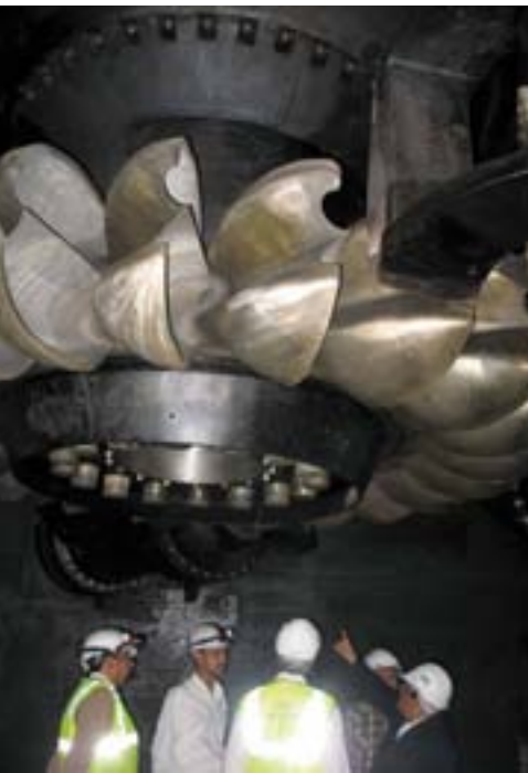
Turbine, Allain Duhangan hydro project, India
